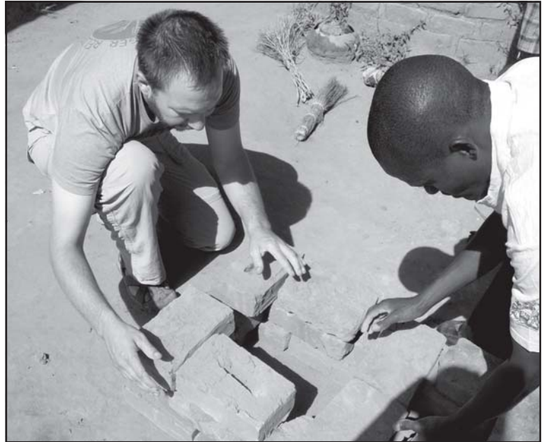
Matt Hess and a Malawian villager construct a wood stove from mud bricks
